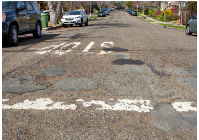
Street Pavement Damage
